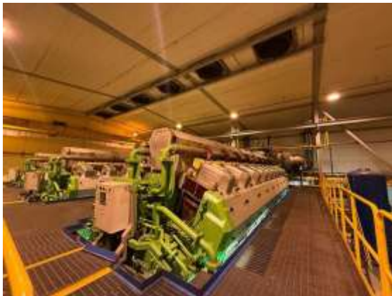
Gambar 2.1 Mesin PLTDG Unit 10,11 & 12 (Sumber: PT. PLN Indonesia power UBP Bali, 2025)
